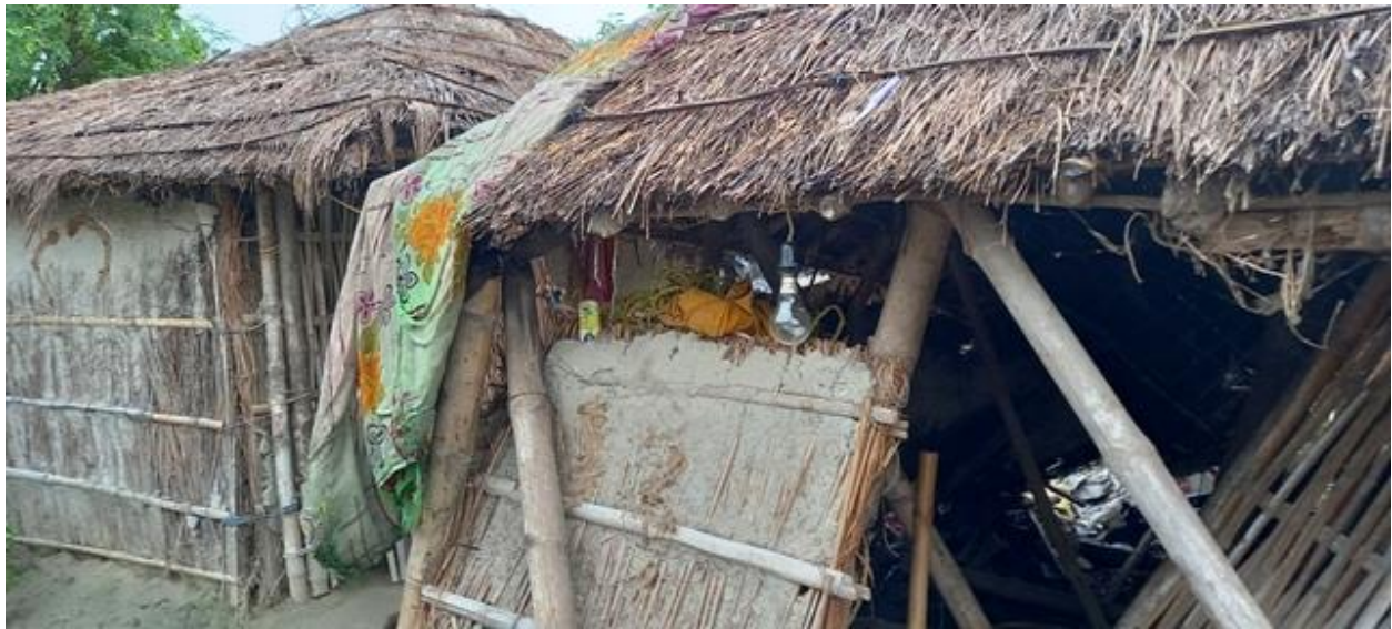
Pic 2.0: By flood damage house
